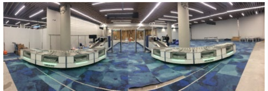
Figure 3: New 'smart lanes' under construction in Auckland International Airport – scheduled for use in November
